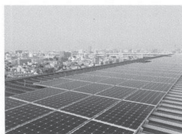
Solar power generation system
